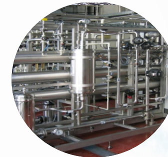
Reverse Osmosis (RO) PLANT
