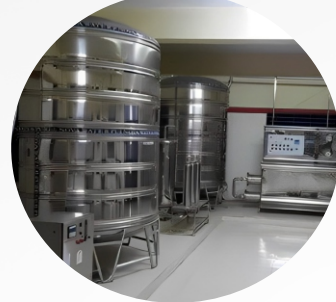
Package Drinking Water Plant
