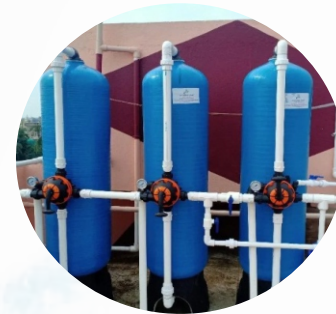
Water Softener Plant
