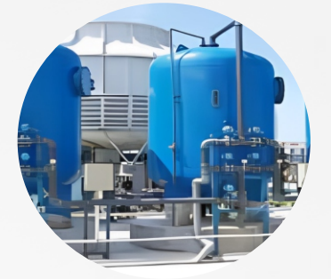
Iron Removal Filter
