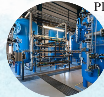
Water Filtration Plant
