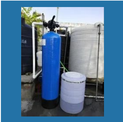
Commercial Water Softening Plant
