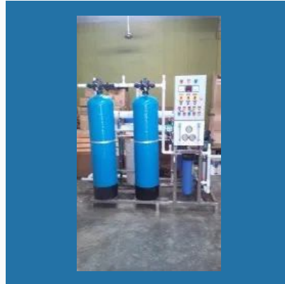
1500 Lph Ro System
