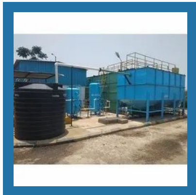
60 kld STP Plant for Biological Treatment
