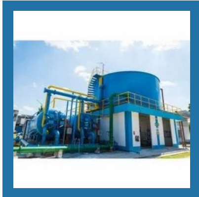
80 KLD STP Plant
