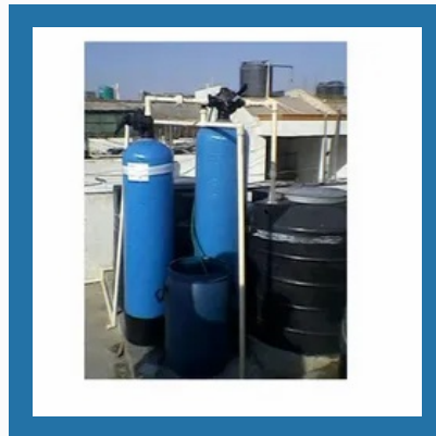
Water Filter & Water Softener Plant
