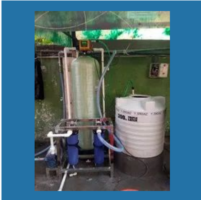
Automatic Water Softener System
