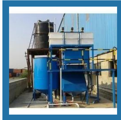
10 Kld Stp Plant
