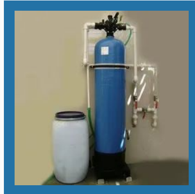
Water Softening Plant
